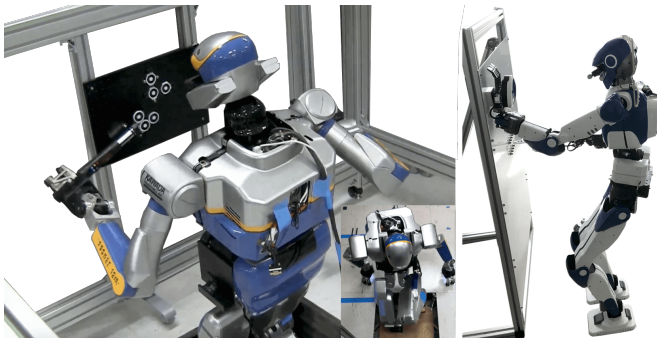
Fig. 14: Narrow access in multi-contact and fast dynamic torquing handling four contacts with HRP-2Kai. (left). Circuit breaker checking combining multi-sensory task-space control with HRP-4, achieved without visual markers (right).
